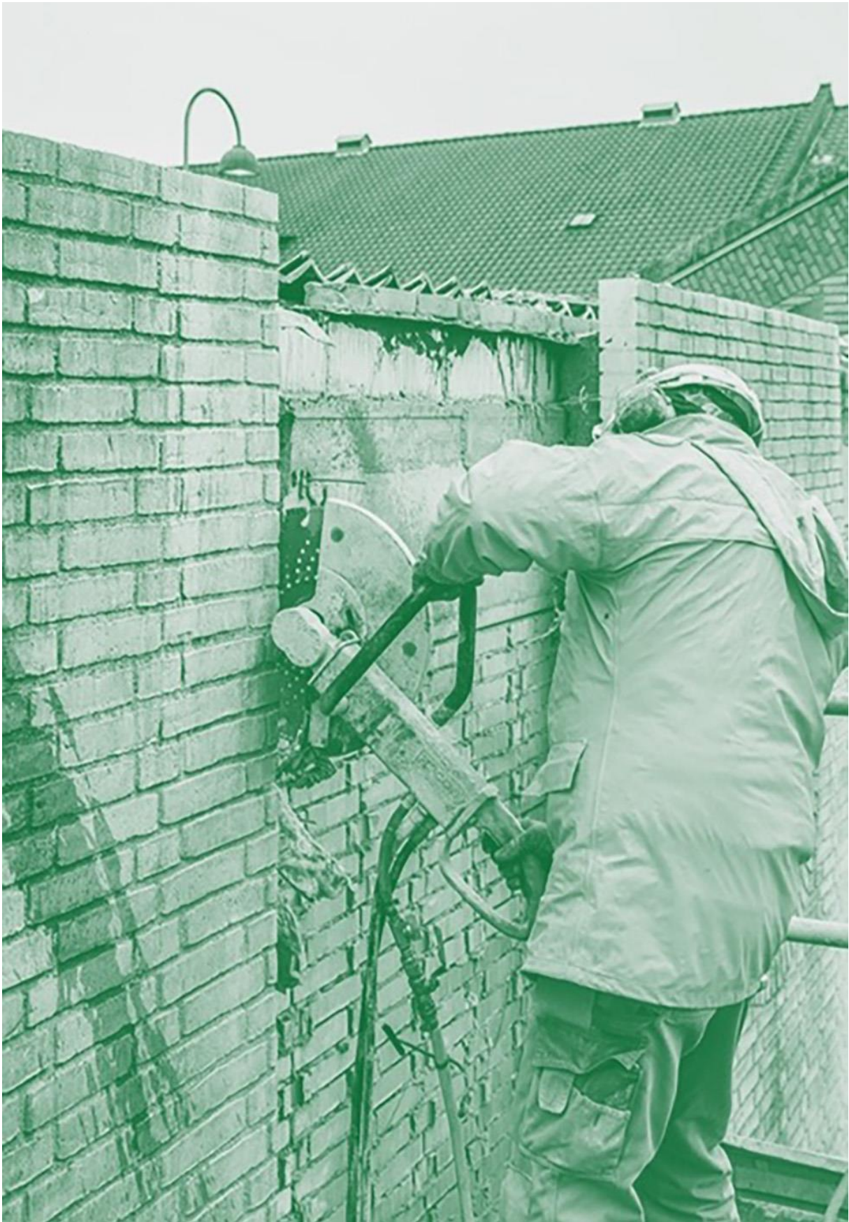
Figure 4: Cutting brick panels to reuse them as façade element, Resource Rows. Photo: Rasmus Hjortshøj.
